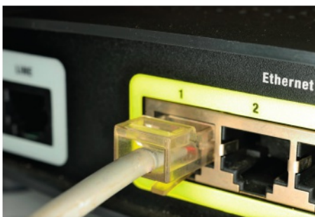
▲ Figure 4.16 An Ethernet connection
