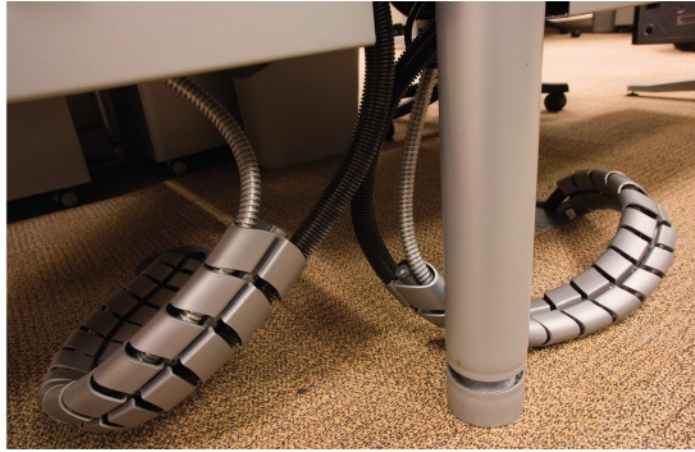
▲ Figure 9.10 Good cable management helps minimise risks to health and safety
