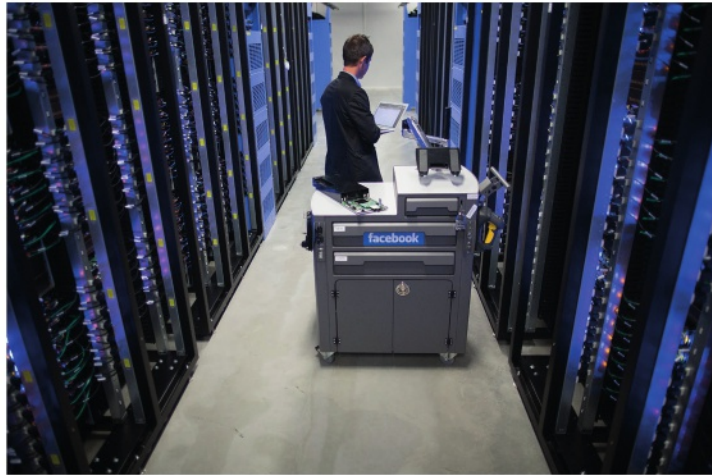
▲ Figure 9.6 Facebook built this data centre in northern Sweden so that it is cooled by Sweden's cold climate rather than an air conditioning system
